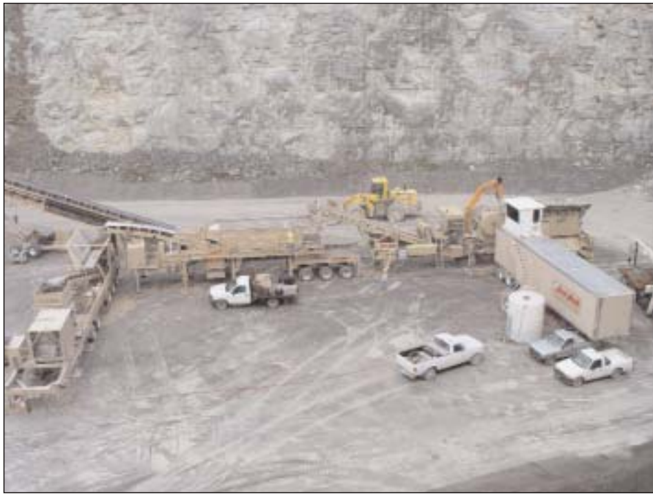
The “front half” of Whitaker Contracting’s Fast Pack plant consists of a Pioneer 3350 Jaw, with a BTI breaker mounted at the grizzly; a JCI 8203 horizontal screen, a Kolberg radial stacker and a JCI K400 Cone Crushing plant.
